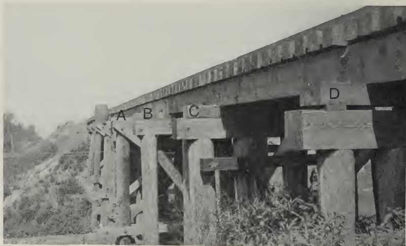
FIG. 40.—Repaired railroad trestle in Franklin County. One end subsided 18 inches more than the other, the total having been reported as about 4 feet. Timbers were placed at A, B, C, and D in order to reduce the sag of the track over the trestle.
